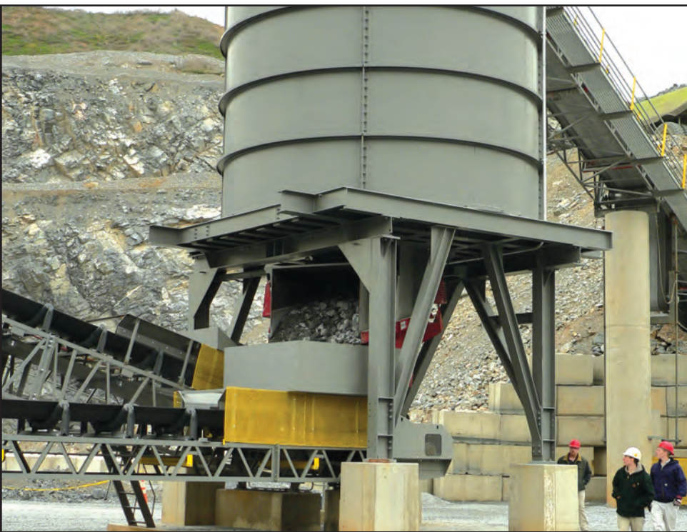
In this unique design, a Syntron Feeder is installed so that it rotates 90 degrees, enabling it to dispense stone onto either of two belts destined for different processing.
