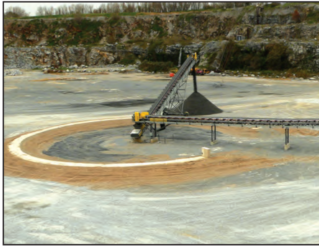
A Steel Systems Equipment-fabricated radial stacker deposits screened aggregate onto a stockpile that can grow to an estimated 50,000 tons in size because of the stackers 270-degrees of travel.
